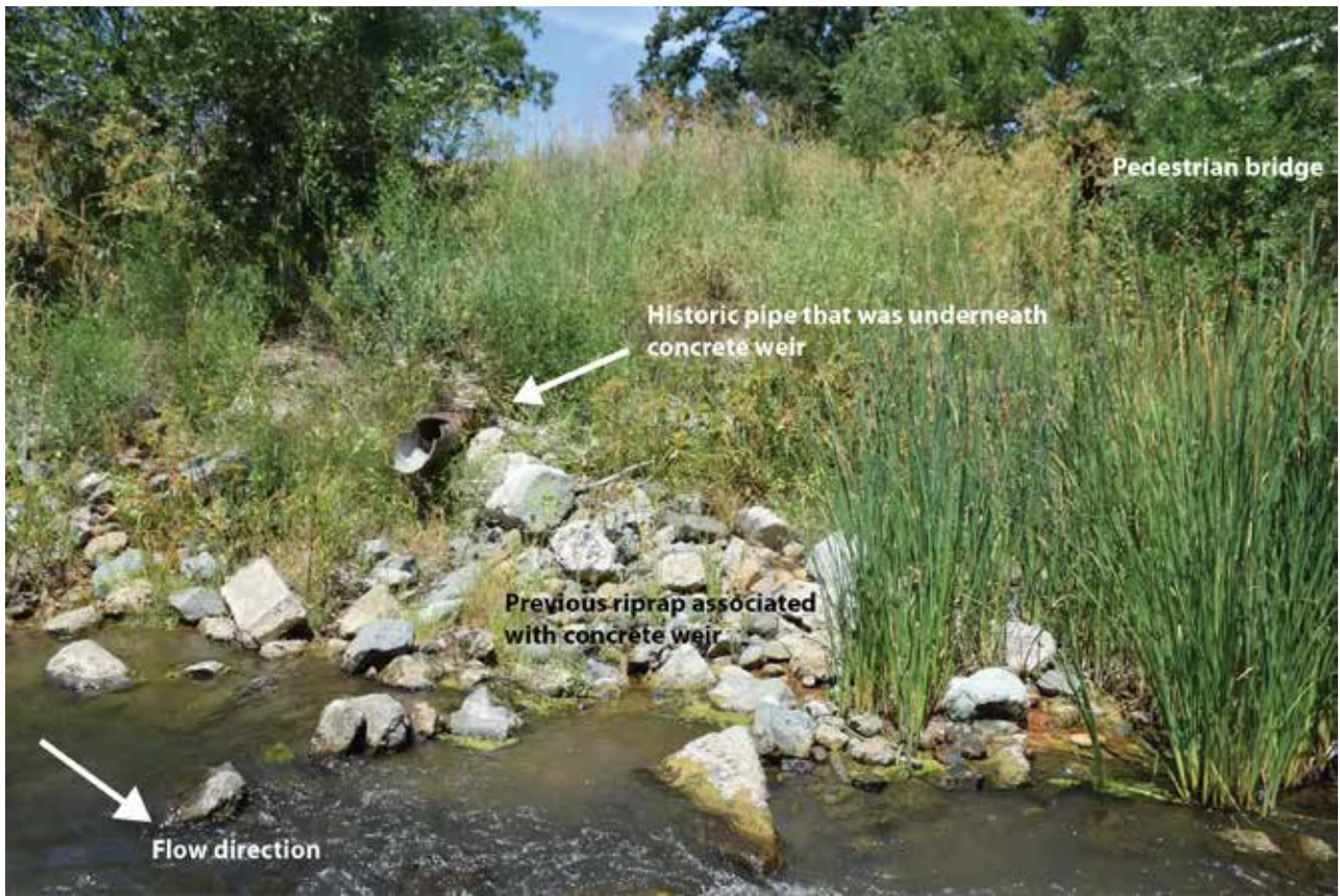
Figure 32. Field photograph of the left bank and an historical pipe that was underneath the concrete weir before it failed and was removed. Pipe is now approximately 1 m above the current bed elevation.
