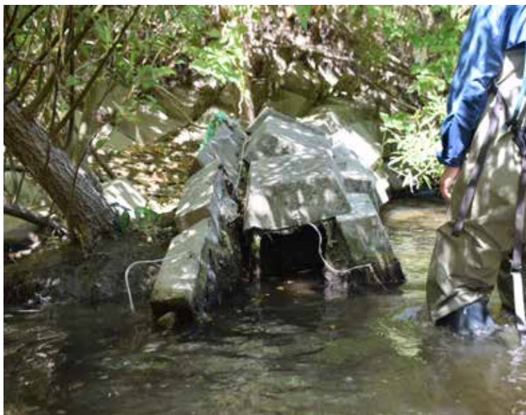
Figure 15. Failing articulated concrete mat.
