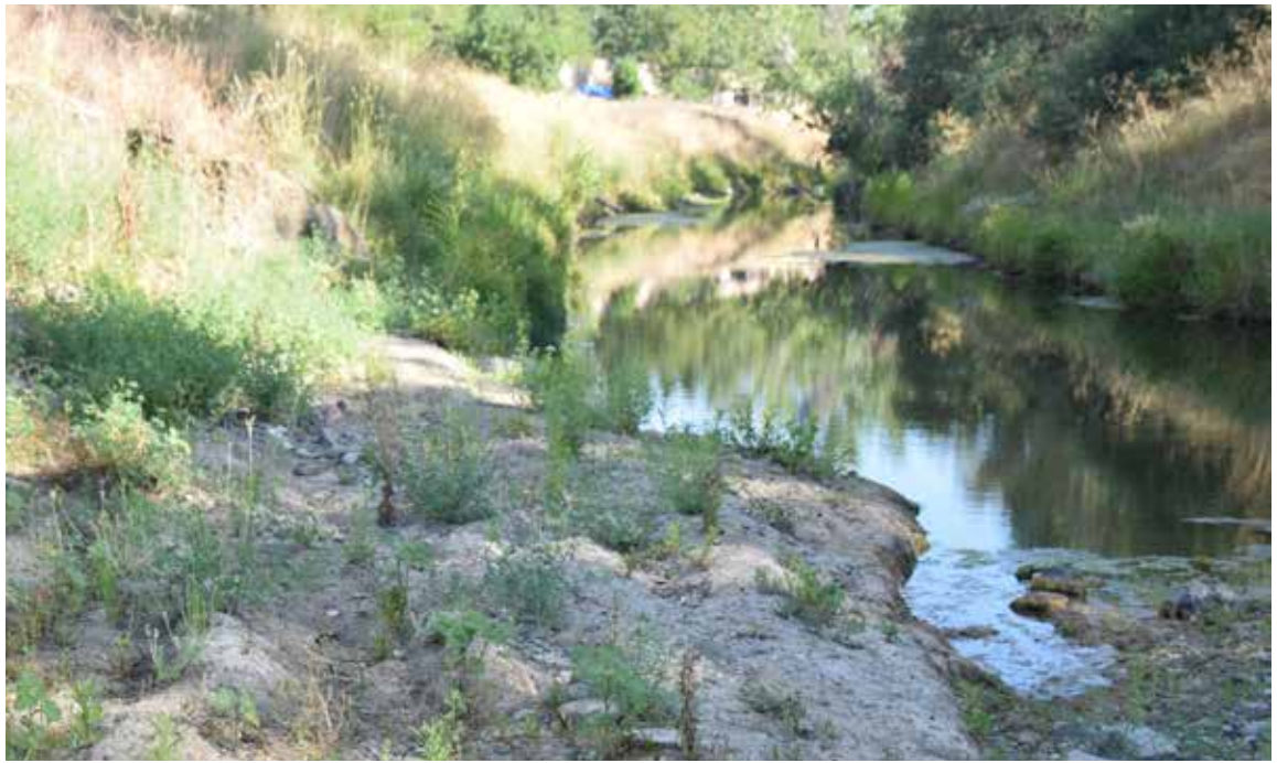
Figure 50. Exposed hardpan on the right bank in the middle of Reach 6.
