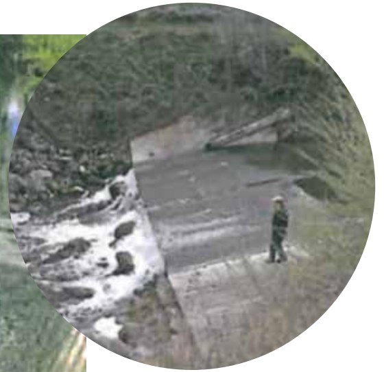
• Figure 31. Two 2007 photos showing the previous condition of the concrete weir before it was undermined and collapsed (courtesy of Zone 7, and Mahacek, 2007).
