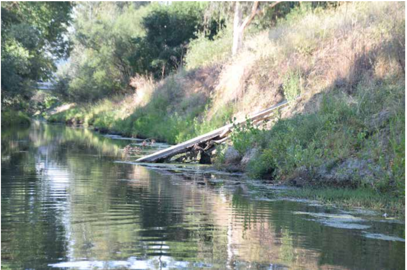
Figure 48. Concrete drain with void space indicating erosion.
