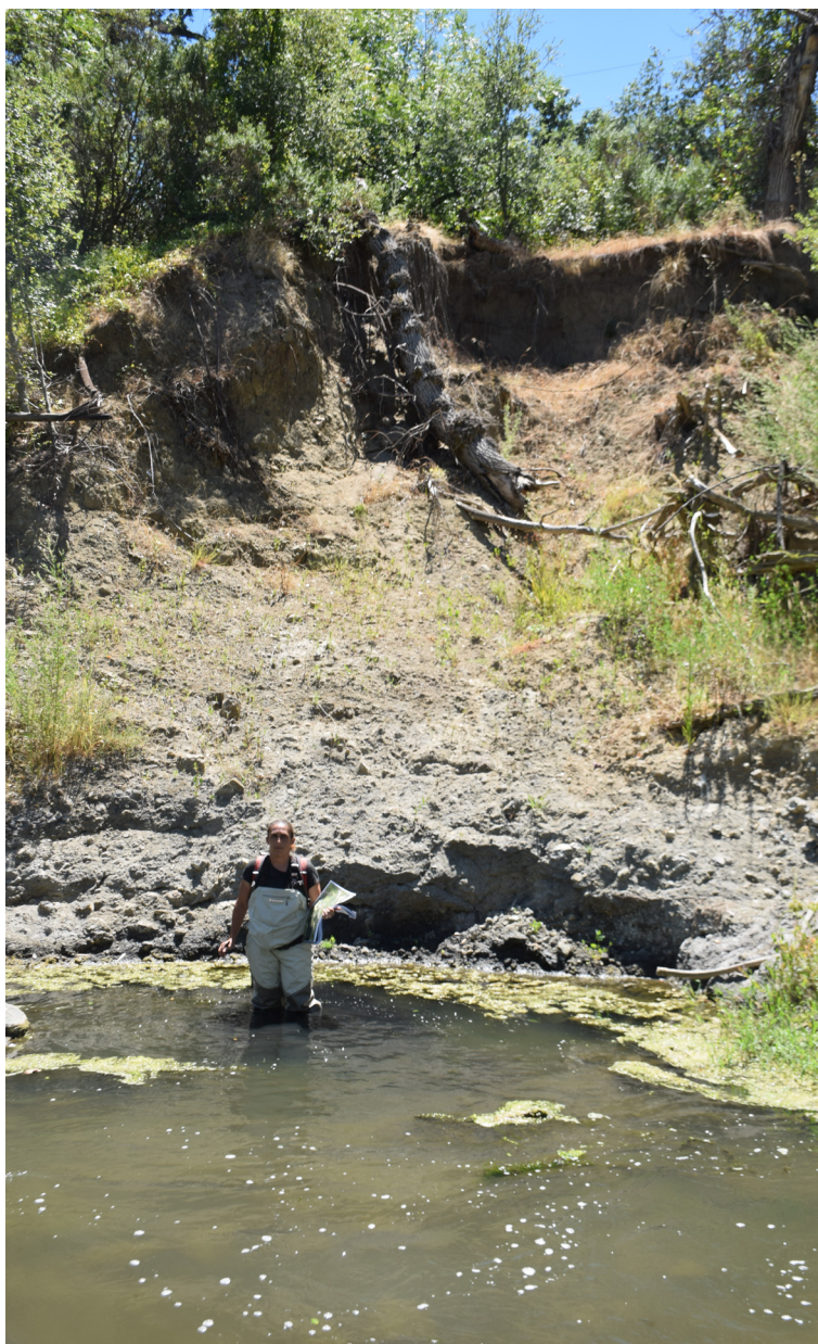
Figure 35. Bank slump location in Reach 4 that is contributing a mix of grain sizes to the channel.
