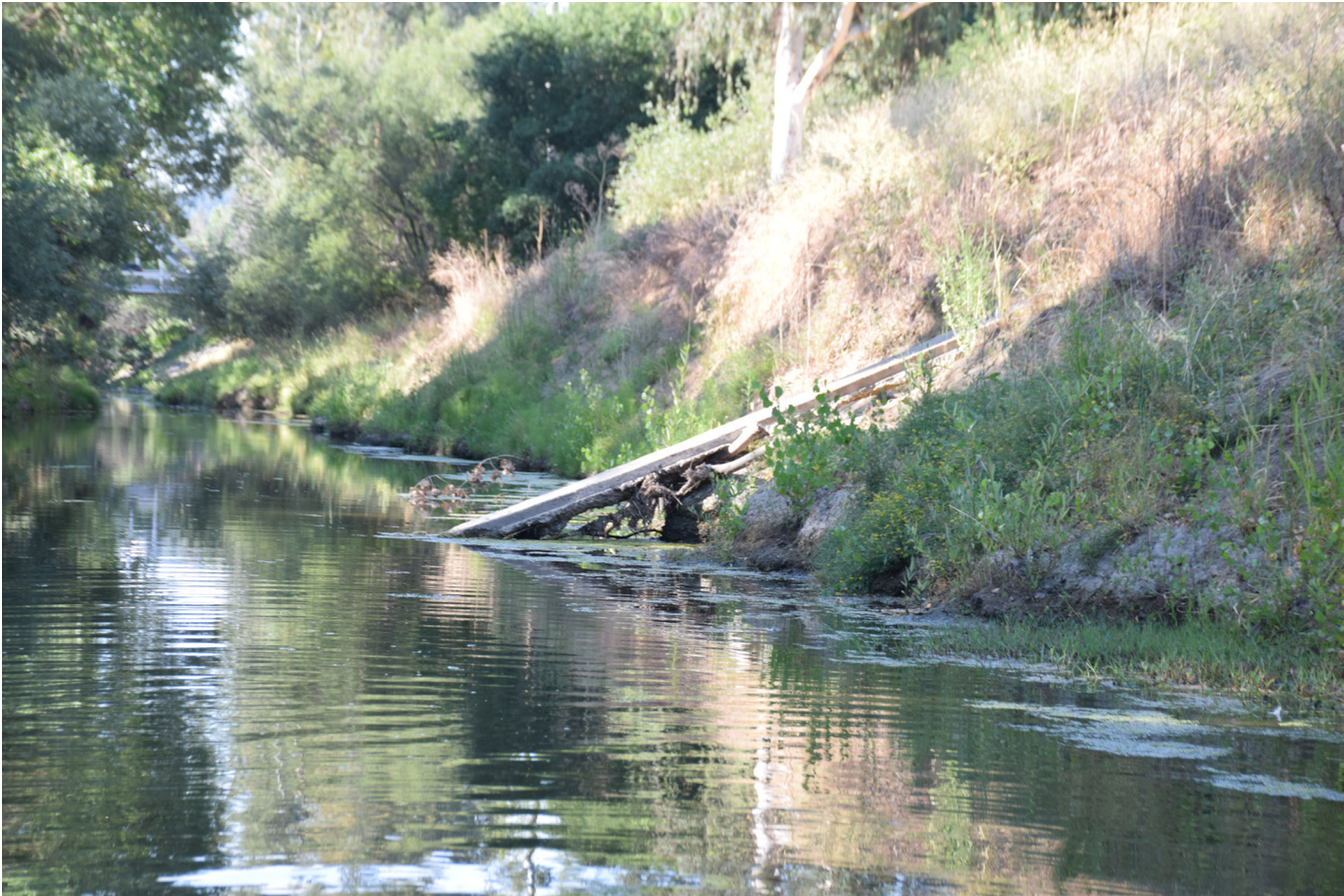
Figure 48. Concrete drain with void space indicating erosion.
