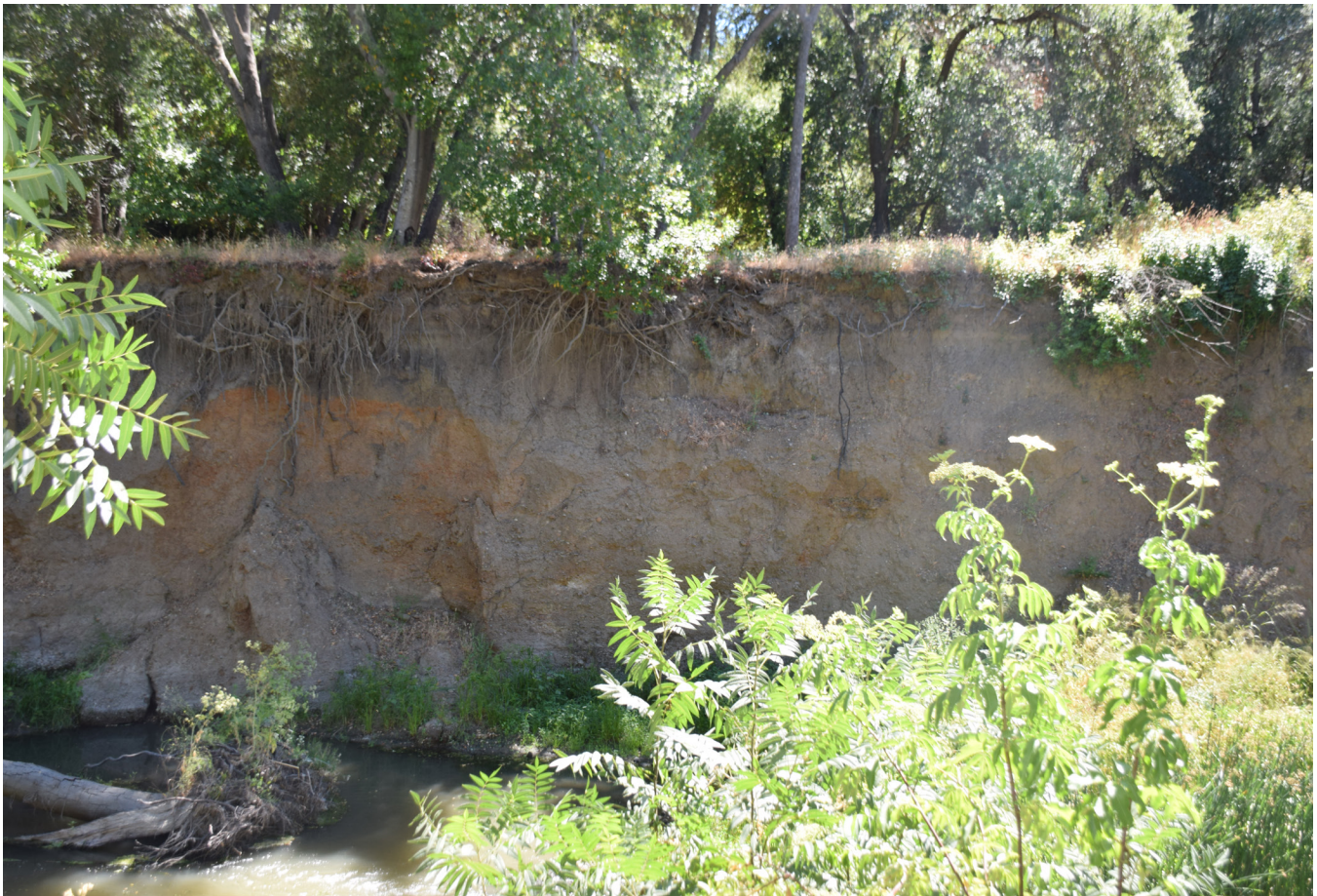
Figure 40. Vertical outer bank and adjacent flat terrace surface (with riparian trees) in Reach 5.
