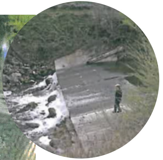
• Figure 31. Two 2007 photos showing the previous condition of the concrete weir before it was undermined and collapsed (courtesy of Zone 7, and Mahacek, 2007).
