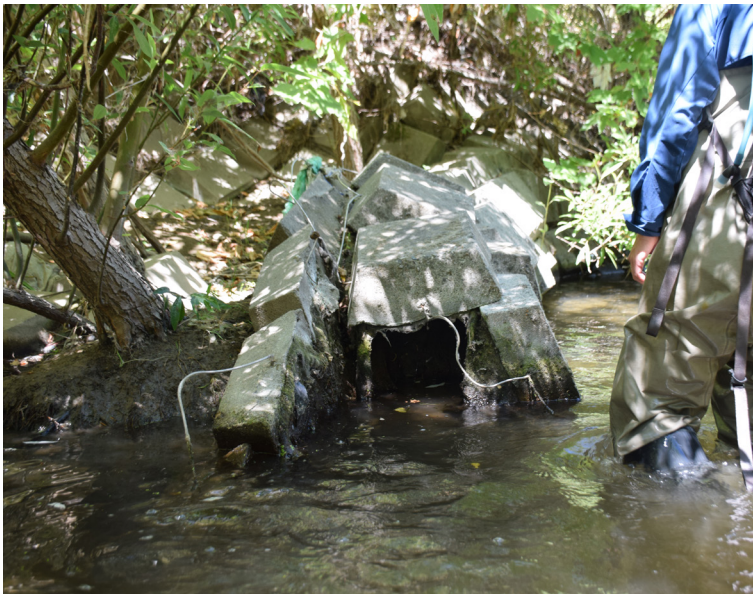
Figure 15. Failing articulated concrete mat.
